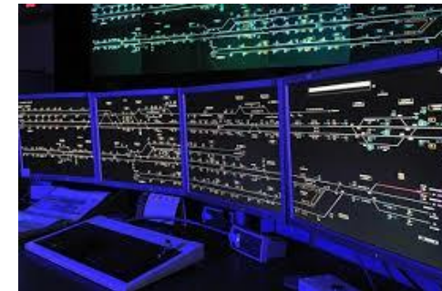
Technology solutions for traffic management, asset management, condition monitoring and passenger Information systems
